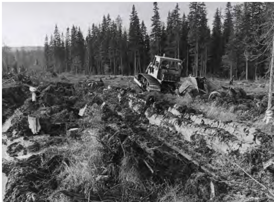
◆ The traces of forest use were shocking in some places. Breaking the soil surface allowed tree seeds to germinate more quickly. In this image a bulldozer is seen pulling a forest plough. Akke Virtanen, the Finnish Forest Industries Federation Collection, Lusto.
