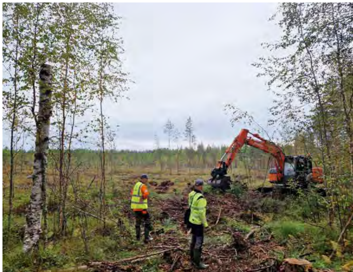
◆ In 2024, Finsilva began the restoration of the Majasuo swamp in South Ostrobothnia by blocking the ditches dug in the 1960s and building dams to raise the water level. Drainage had failed, and no trees had grown on the swamp. Restoration has enhanced the biodiversity on the dried swamp and improved the condition of nearby water bodies. Finsilva.
